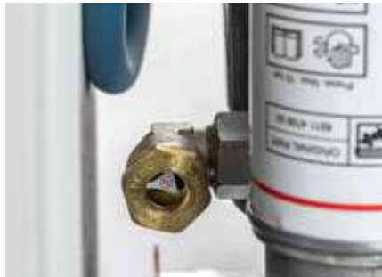
/// Oil level check
